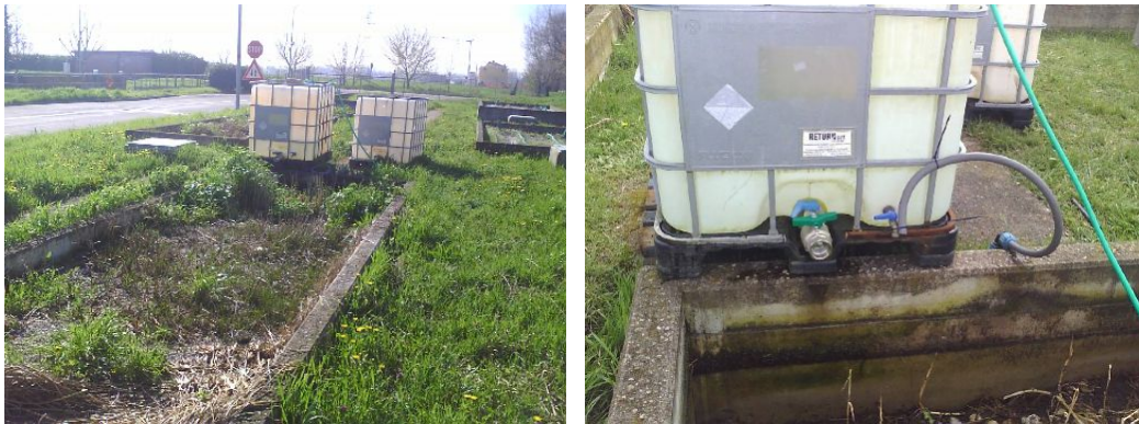
Figure 4.27.: Ferrara H-SSF pilot plant for the second investigation
